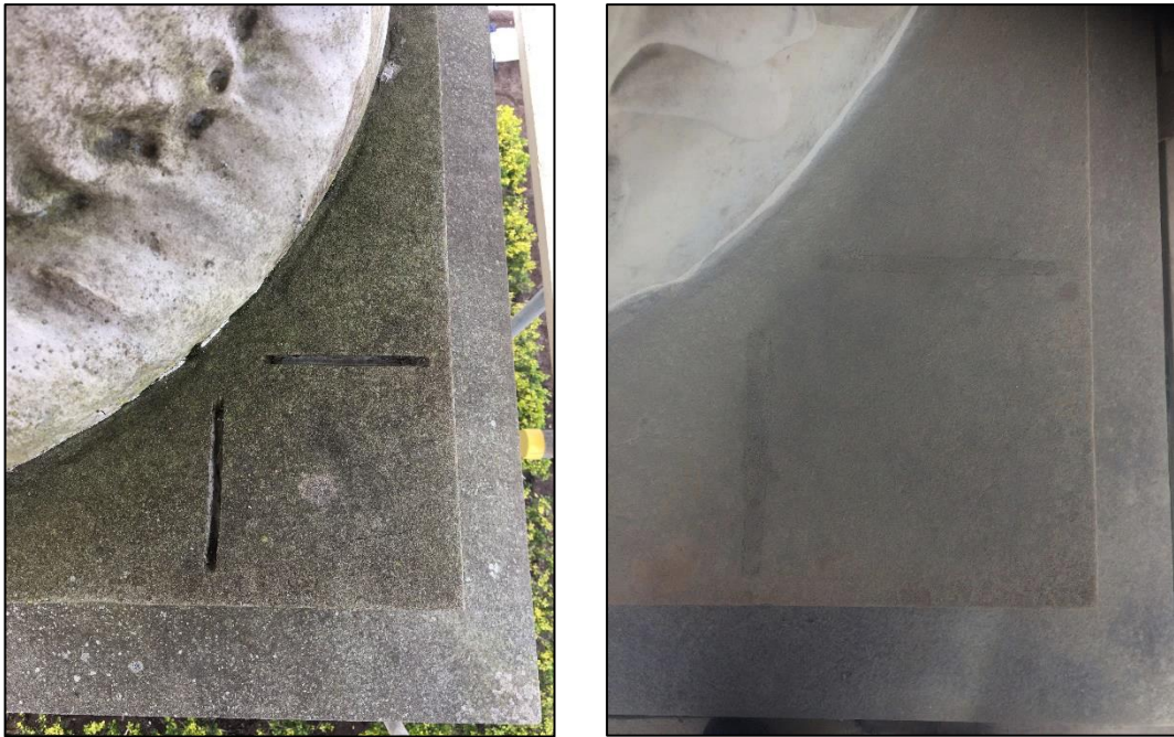
Metal cramps set into channels at the top of the sandstone plinth before (left) and after (right) polyester resin and Paraloid B72 repair
