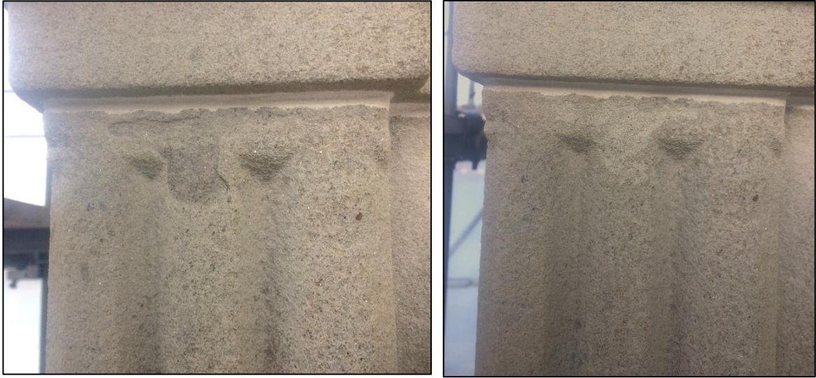
Surface scaling to triglyph moulding before (left) and after (right) Paraloid B72 repair
