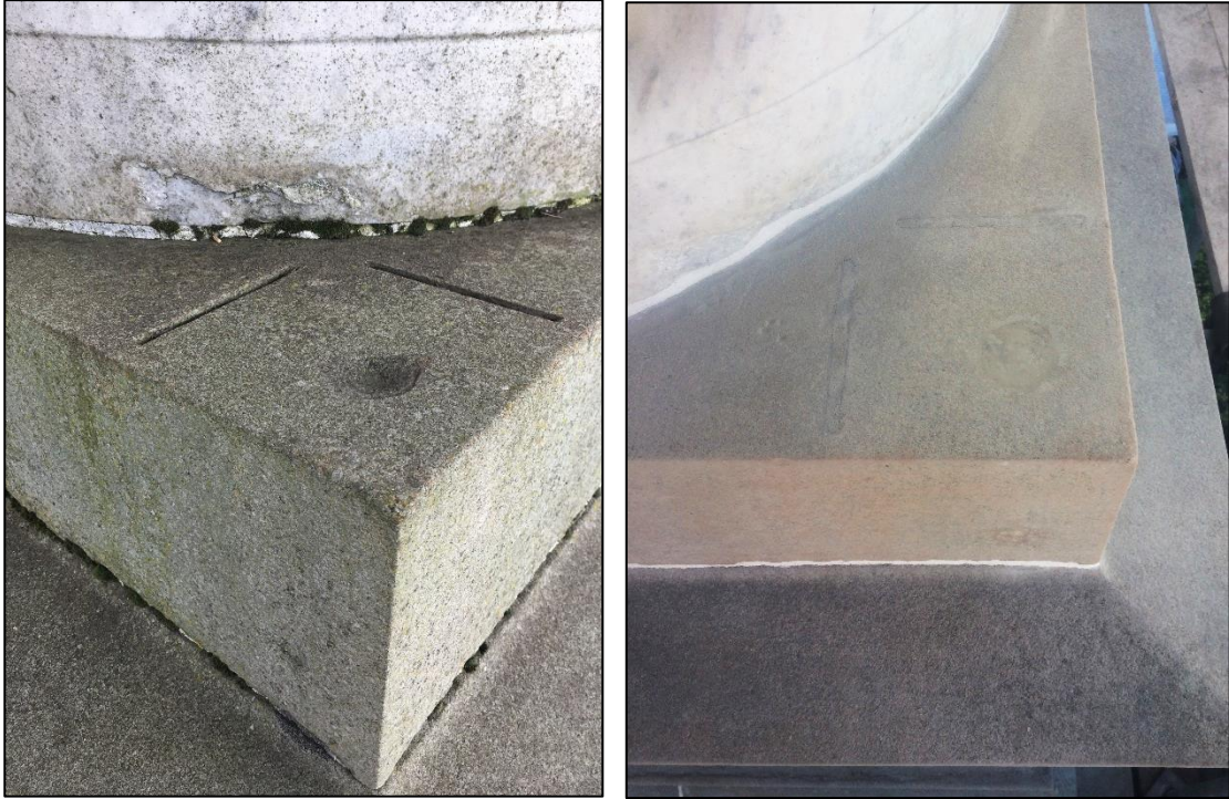
Metal cramps set into channels at the top of the sandstone plinth before (left) and after (right) polyester resin and Paraloid B72 repair. Circular loss before (left) and after (right) Paraloid B72 repair
